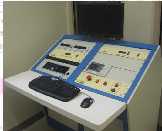
ASD Controller & Control Panel
